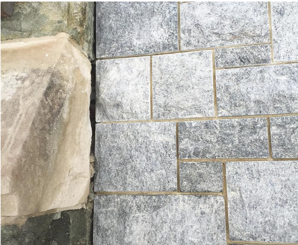
To help with the placement, each piece of stone had a specific stonemark and piece number so once the stones were ready to be placed, it would be easier to determine where each stone belonged. Photo courtesy of Coldspring
