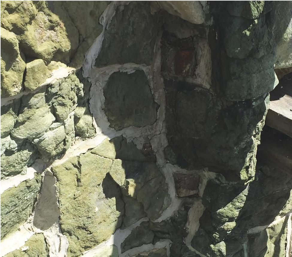
To pay tribute to the parish's Irish heritage, the original builders selected green serpentine for its exterior but that decision would prove to be an issue 100 years later when the existing serpentine had deteriorated and safety had become a concern. Photo courtesy of Coldspring
